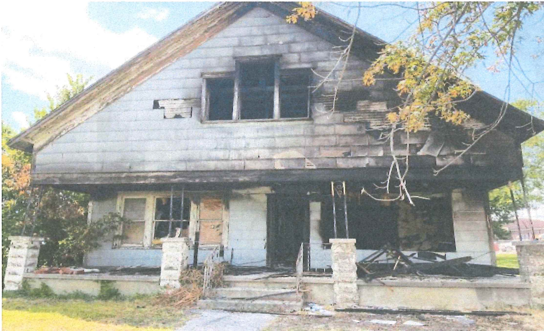
@ 1,854 square feet single level dwelling. Recent fire.
