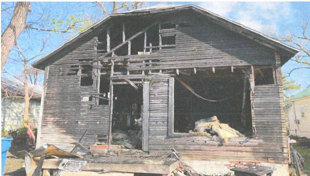
@ 874 square feet single level dwelling. Recent fire.
