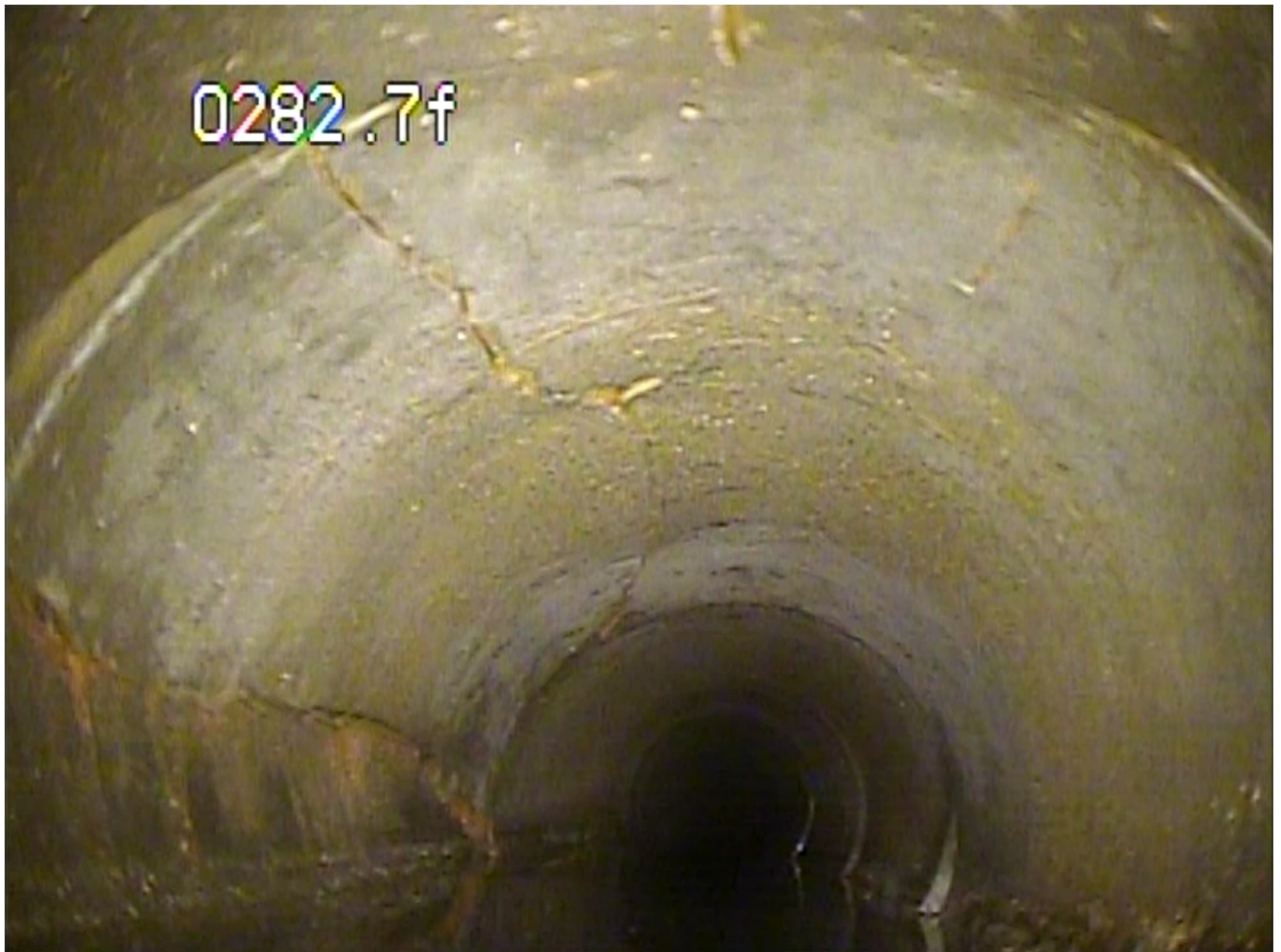
Segment MH 4-5 to MH 4-6: Cracking
