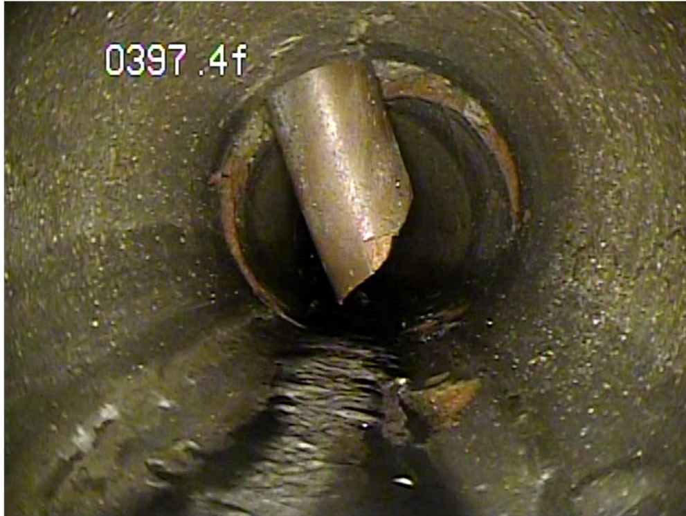
Segment MH 4-2 to MH 4-3: Intruding Tap
