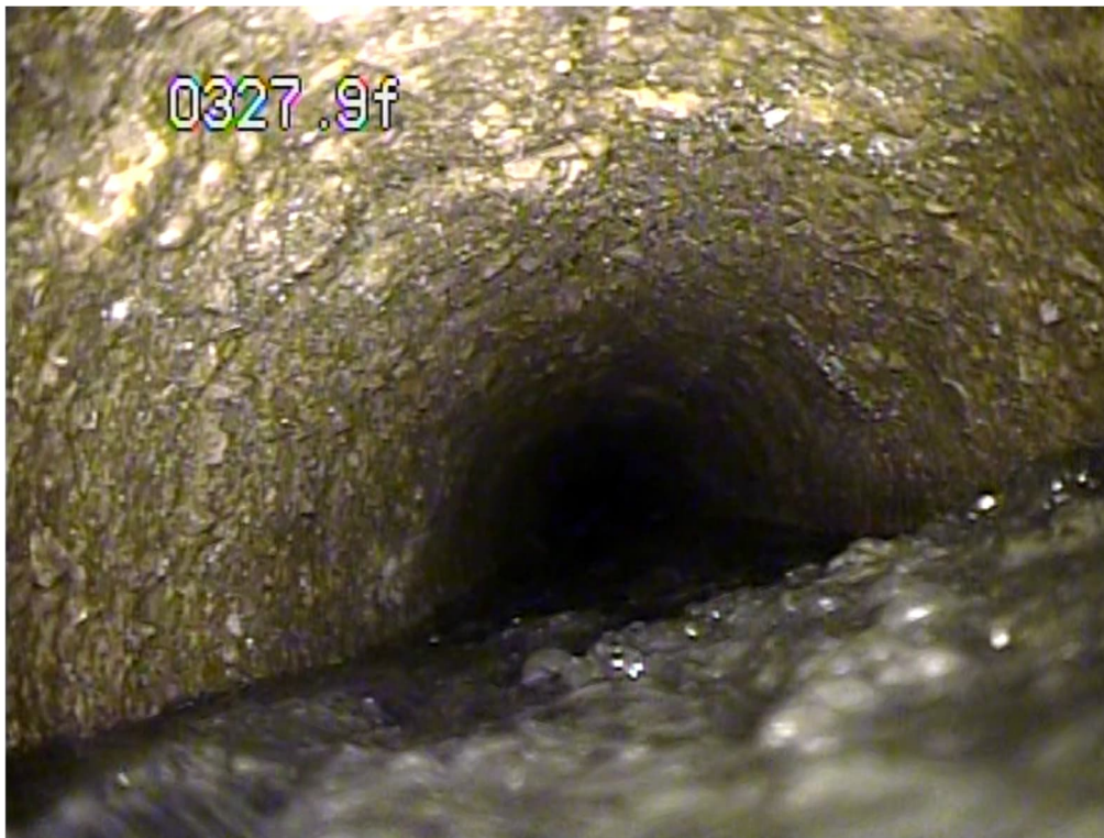
Segment MH 4-18 to MH 4-1: Sediment Deposit
