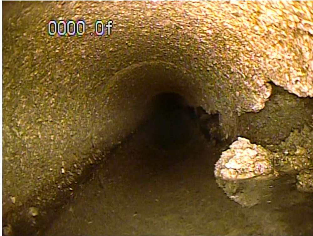
Segment MH 4-18 to MH 4-1: Missing Pipe Wall.
