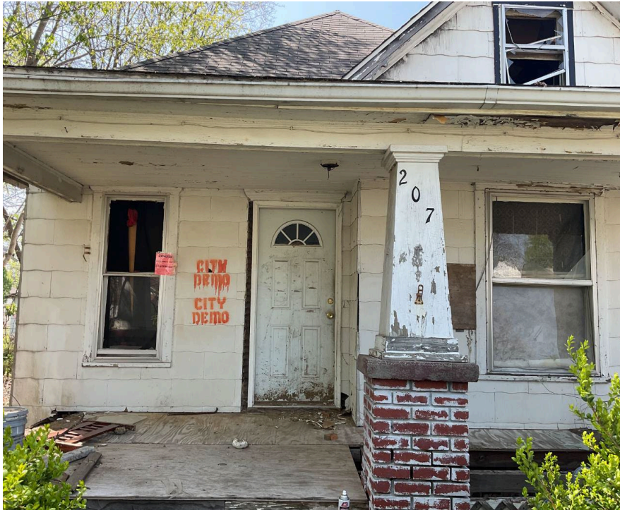
207 W. 2 nd Street- Structure Fire- 1 story 1,126 Sq./Ft. & shed 264 Sq./Ft.
