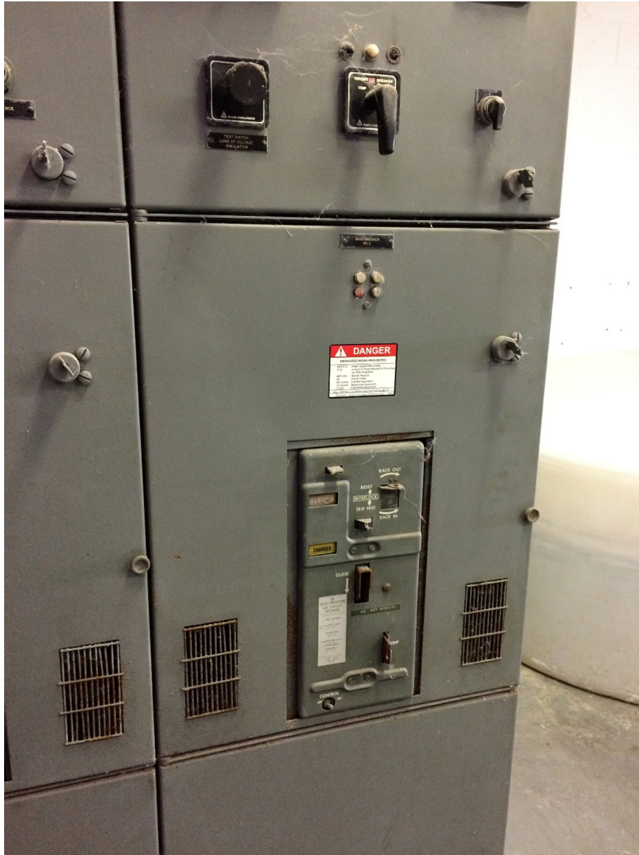
800 Amp Main Breaker 2 (Right Bucket)
