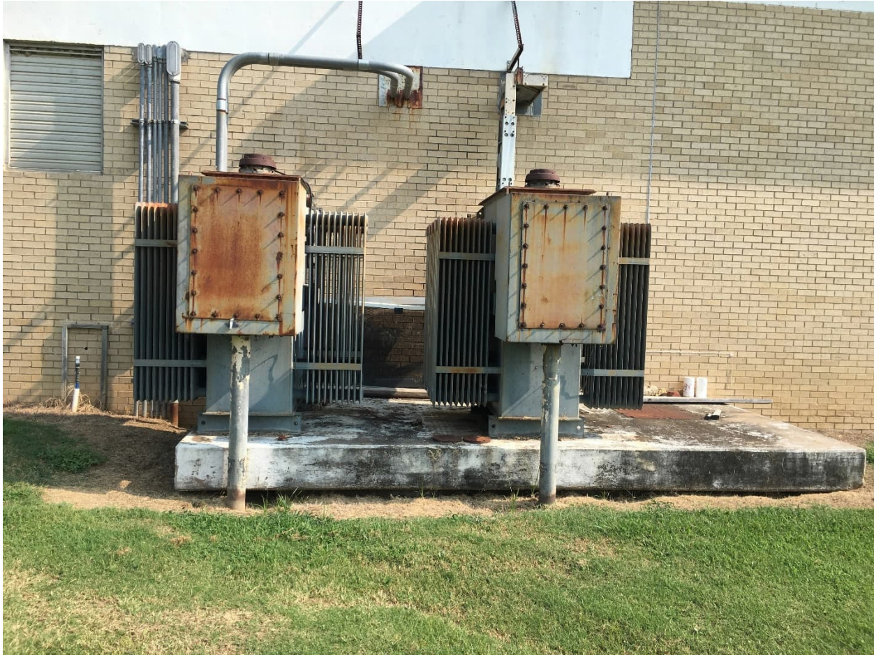
1000 kVA Pad Mount Transformers
