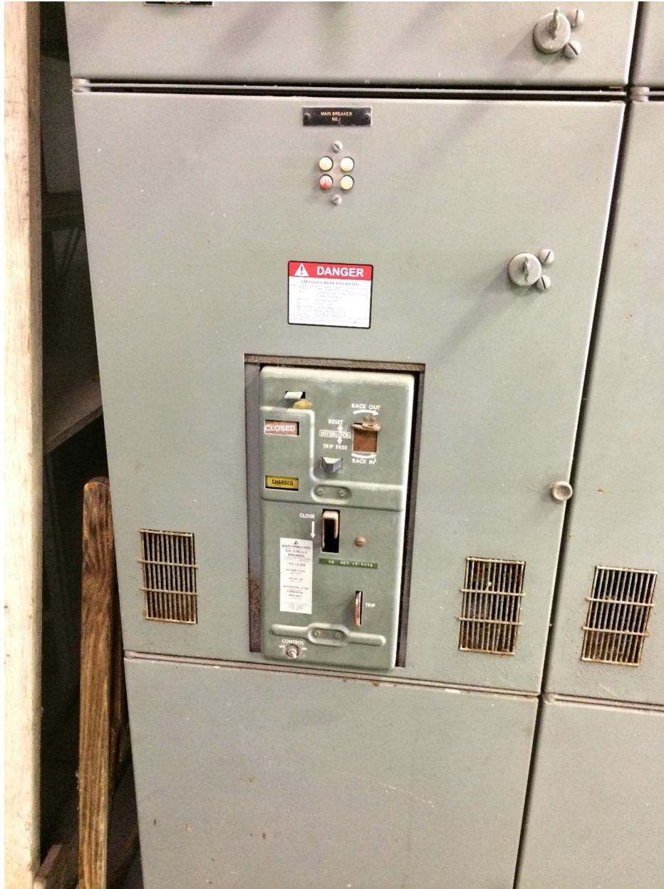
800 Amp Main Breaker 1 (Left Bucket)
