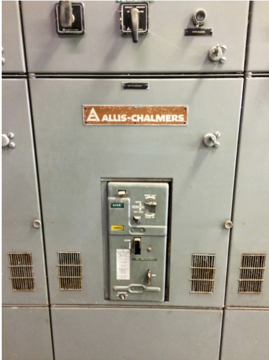
1600 Amp Main Tie-Breaker (Center Bucket)
