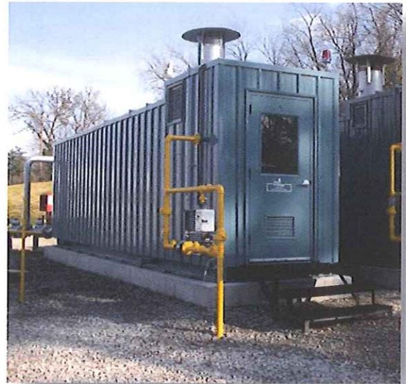
Figure 1: Example Heater with Maintenance House
