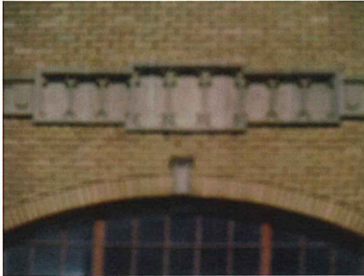
MASONRY JOINT CRACKING.
