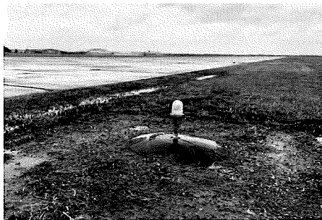
Existing Runway Light With Protection Ring
